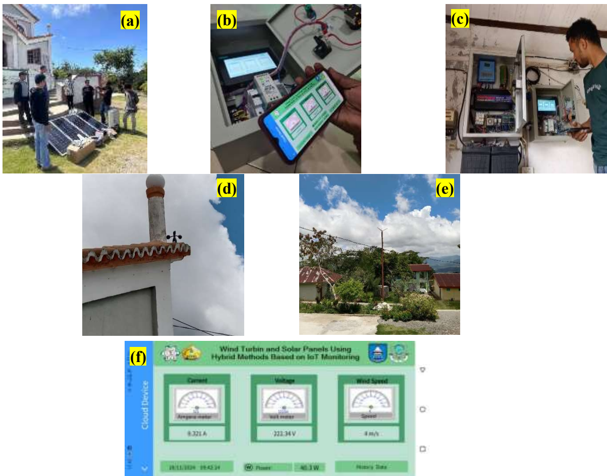
Figure 3.1 Instalation hybrid system at the location (a) Solar Cell (b) Electrical Control panel box and IoT panel box (c) Position control box in the Church (d) Anemometer position (e) Wind Turbine Position (f) IoT system monitoring use Haiwell Cloud
